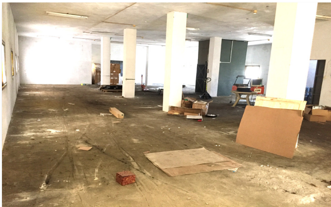
The building in Nazareth in need of renovation
